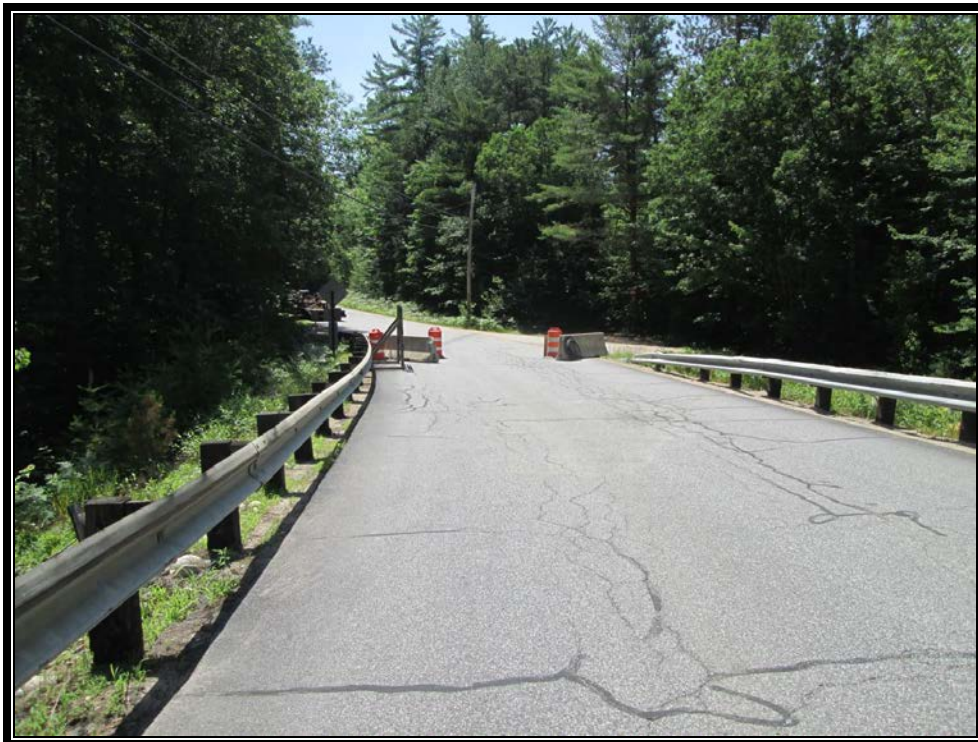
Photo 1: Road closed sign and jersey barriers at south approach.
