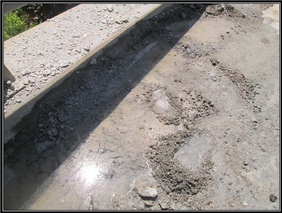
Photo 3: Deteriorated concrete along curb line.
