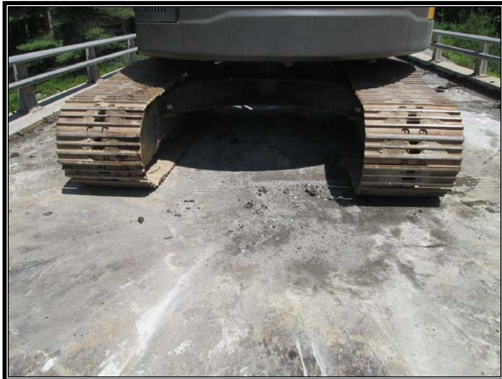
Photo 5: Isolated location of deteriorated concrete in middle of deck.
