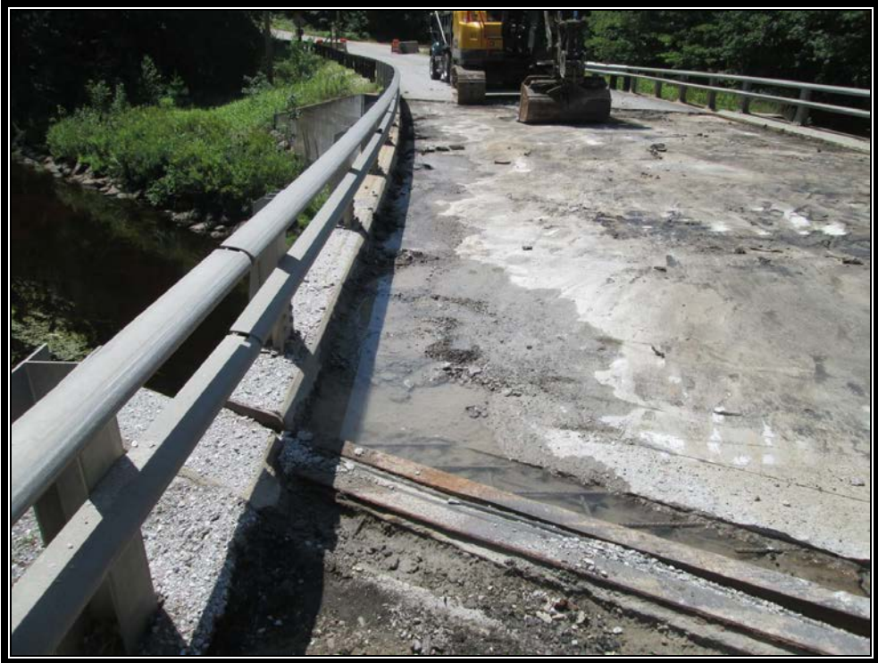
Photo 2: Pavement removed on bridge deck. Note deteriorated deck pavement along curb and backwall
