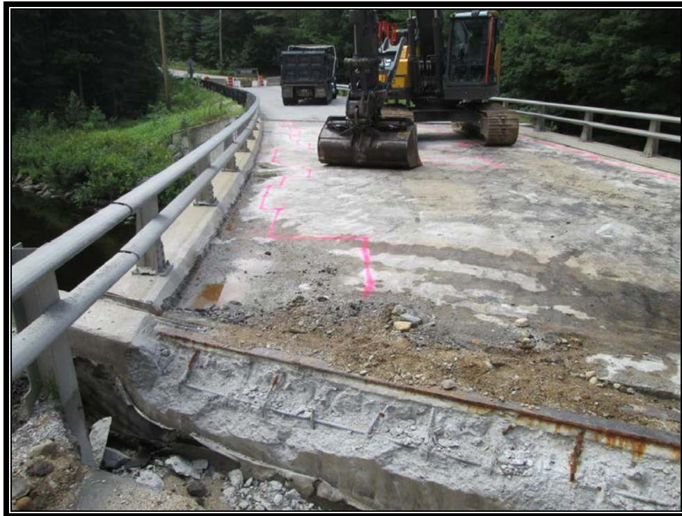
Photo 1: Marked locations for deck repair along the east curb line.
