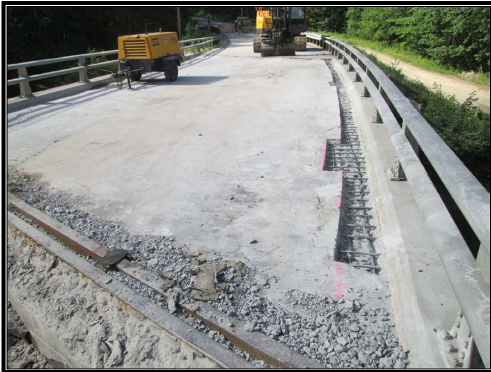
Photo 1: Concrete deck chipped out along the west curb.
