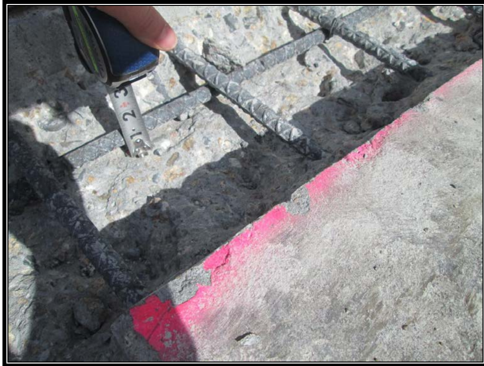
Photo 2: Exposed reinforcing steel along the west curb.
