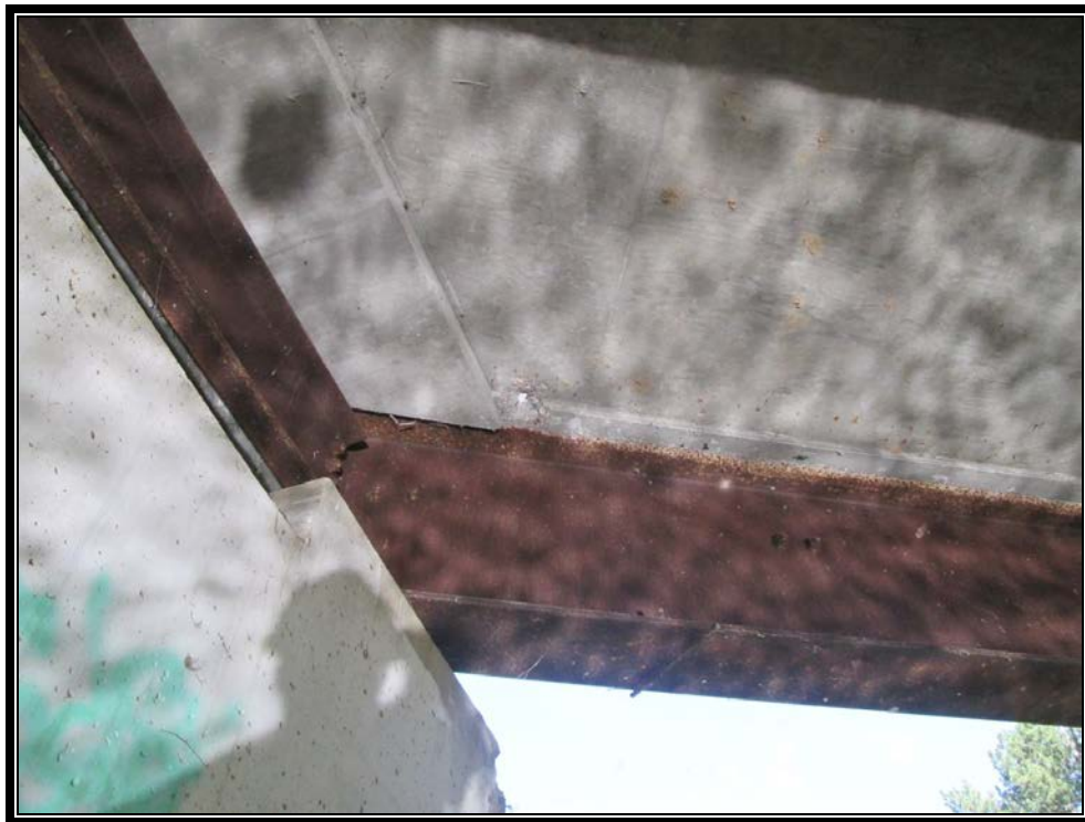
Photo 3: Spall at bottom of deck where Contractor broke through.
