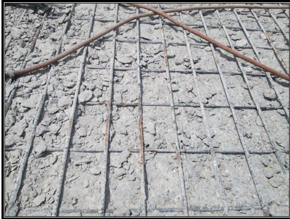
Photo 2: Reinforcing steel with section loss.
