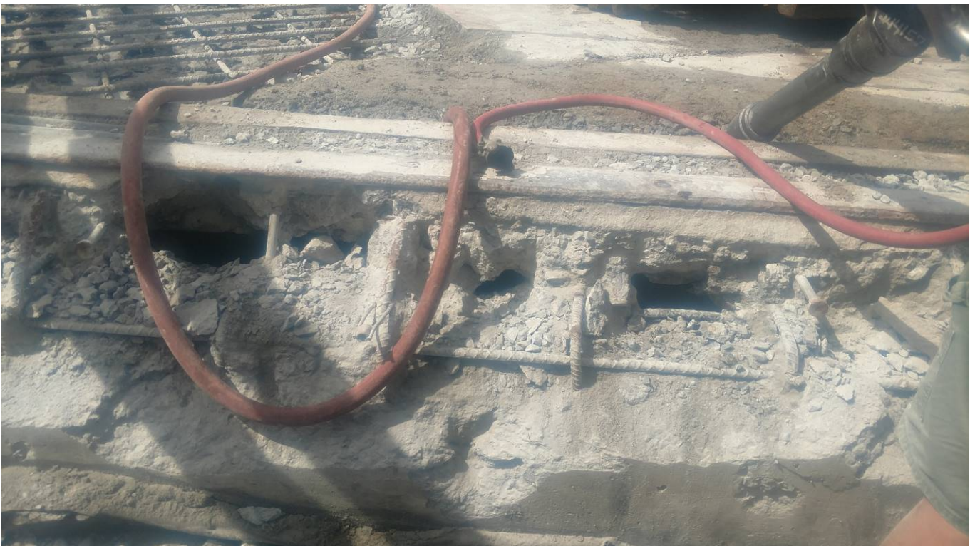
Photo 3: Hole below expansion joint in backwall.
