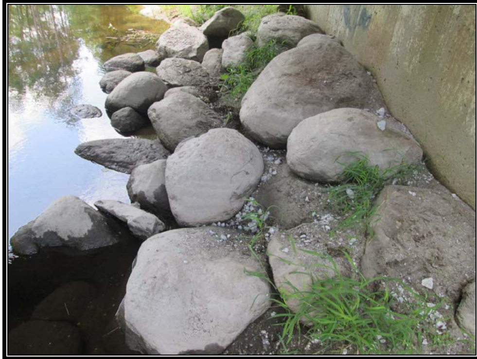
Photo 4: Concrete debris along the riverbank and in the river.
