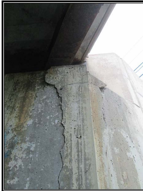
Photo 5: Loose concrete at the north abutment.
