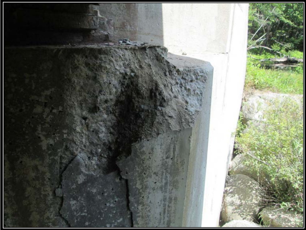
Photo 4: Deteriorated concrete behind location of loose block.
