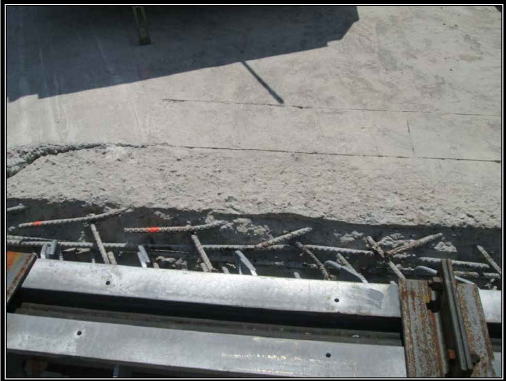
Photo 5: Deteriorated concrete at end of deck.
