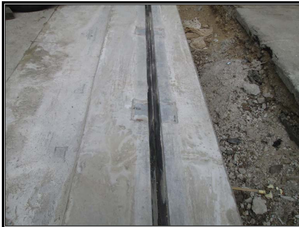
Photo 2: Rough concrete and welds to be grinded clean.
