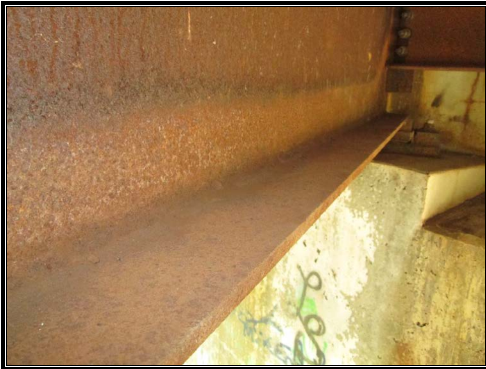
Photo 1: Girder with loose rust removed.
