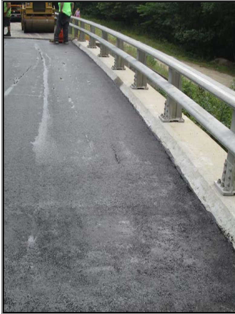
Photo 4: Bubble in membrane translating through pavement at north end of bridge.
