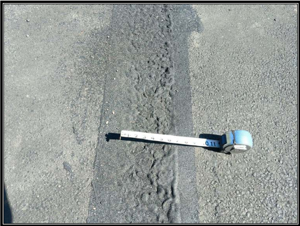
Photo 2: 6-inch-wide plug joint.
