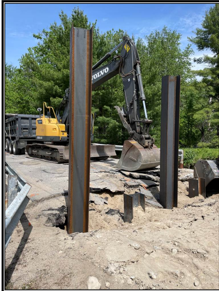
Photo 1: Large stones/debris inhibit the end piles on the east side
