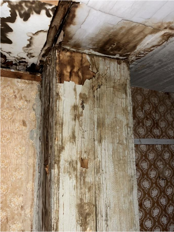
21 Town House Road, Center Effingham Ell Chimney severe disrepair FIRST FLOOR (TOP) THIRD FLOOR
